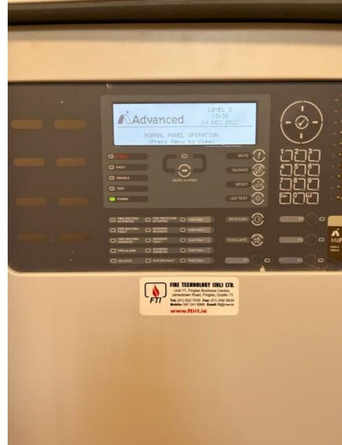
Fire Alarm Panel
