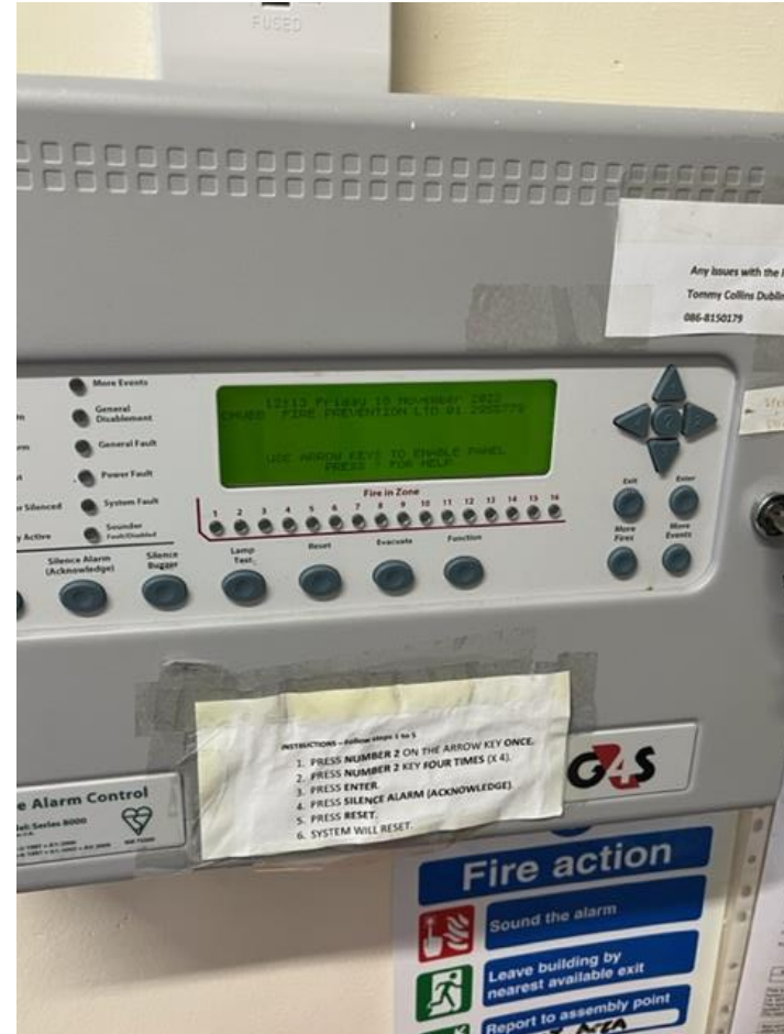
Fire Alarm Panel
