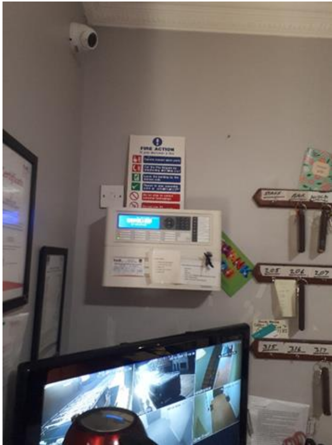
Fire Alarm and CCTV
