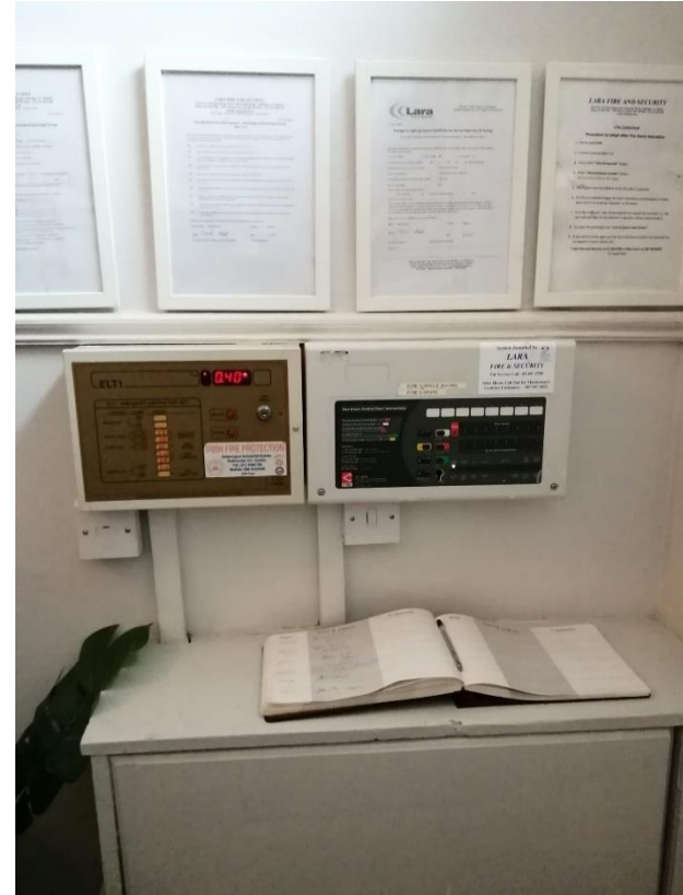
Fire Alarm Panel
