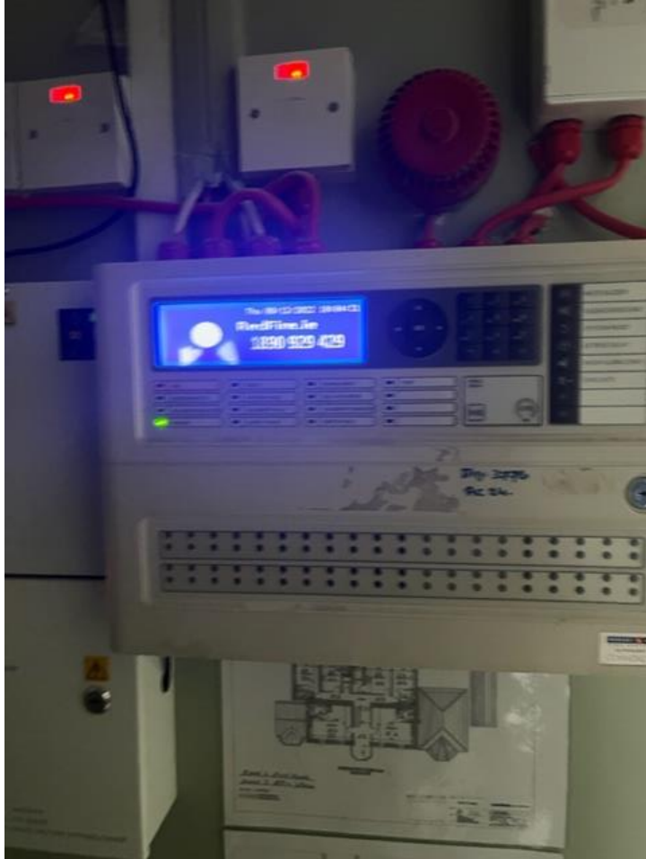
Fire Alarm Panel
