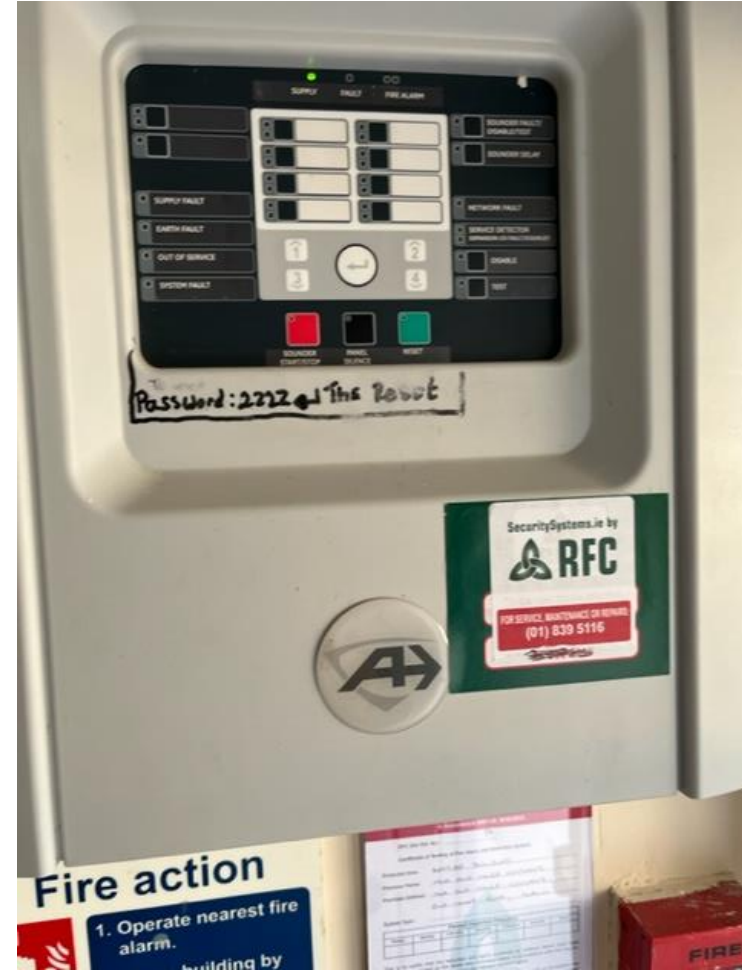
Fire Detection Alarm
