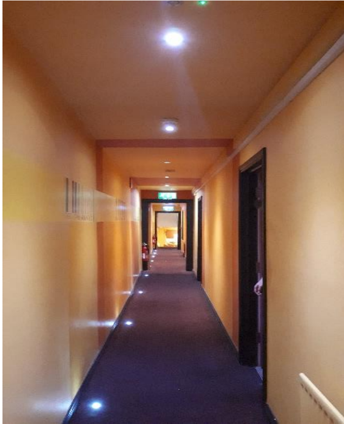
Emergency Lighting/ Fire Extinguisher
