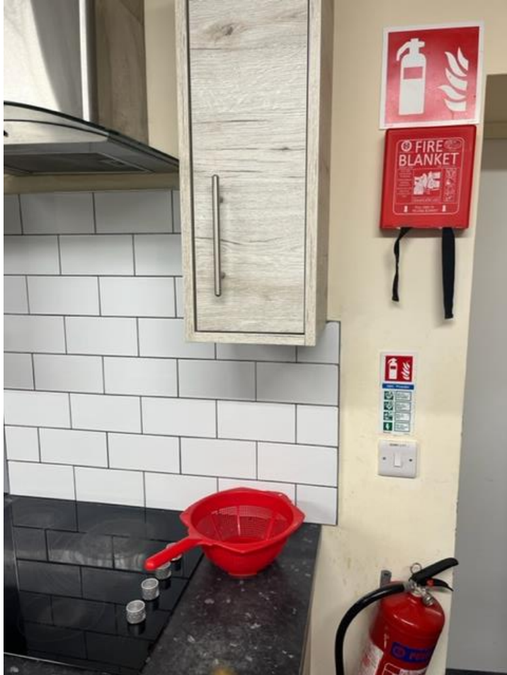
Kitchen Fire Safety
