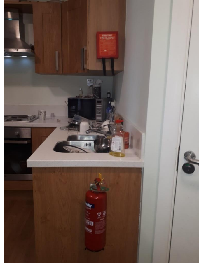
Blanket and Extinguisher in each bedroom
