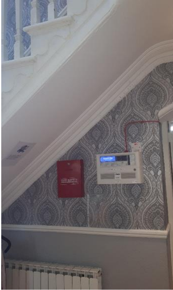
Reception/Fire Alarm System
