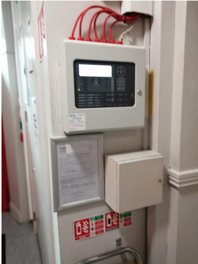
Fire Alarm System
