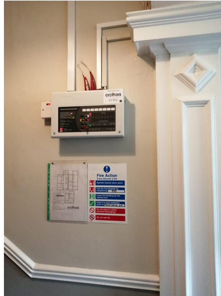
Fire Alarm Panel
