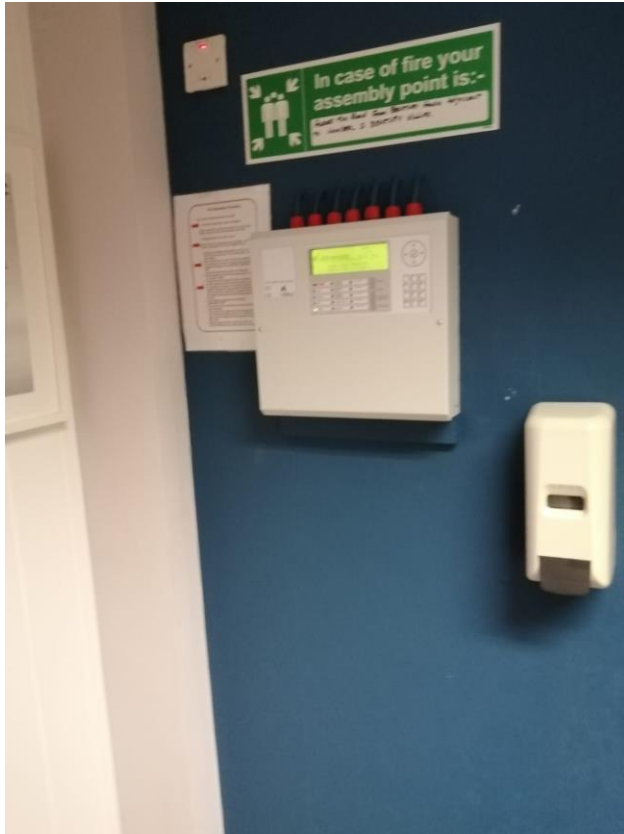
Fire Alarm System
