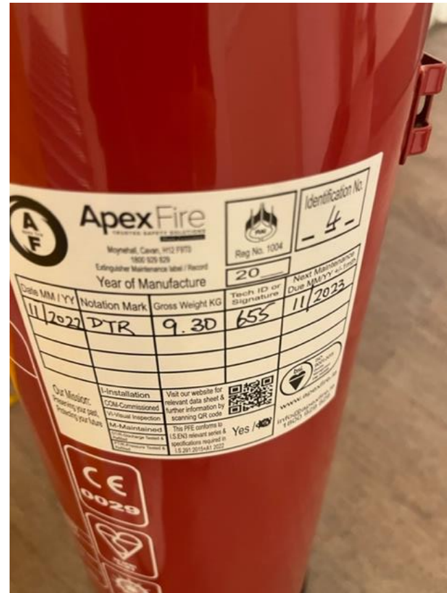
Fire Extinguisher serviced
