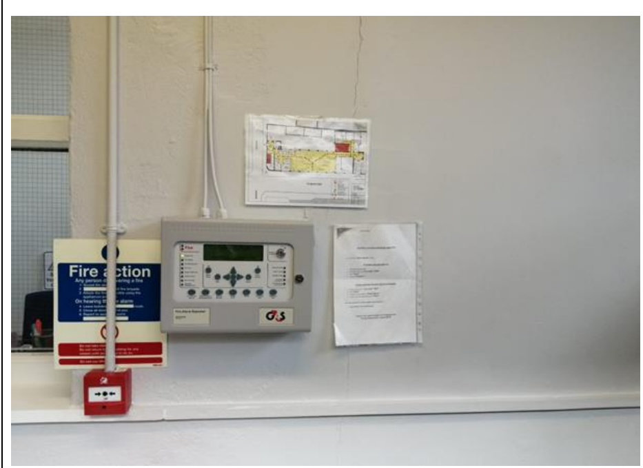
Fire Alarm System
