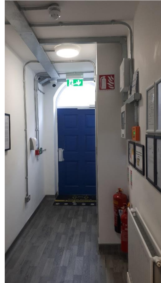
Fire Points, Emergency Lighting
