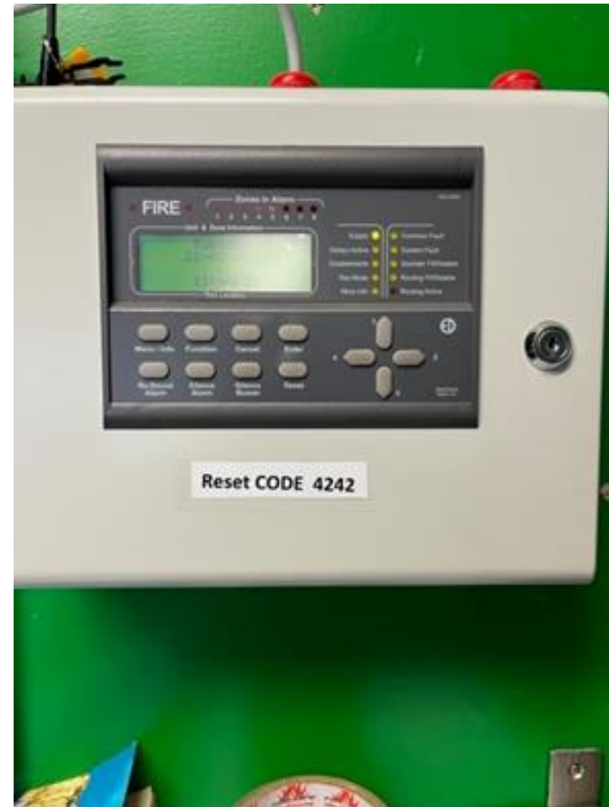
Fire Alarm Panel
