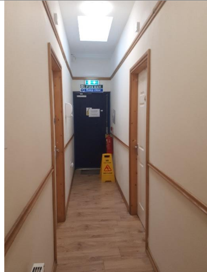
Fire Extinguishers /Emergency Lighting
