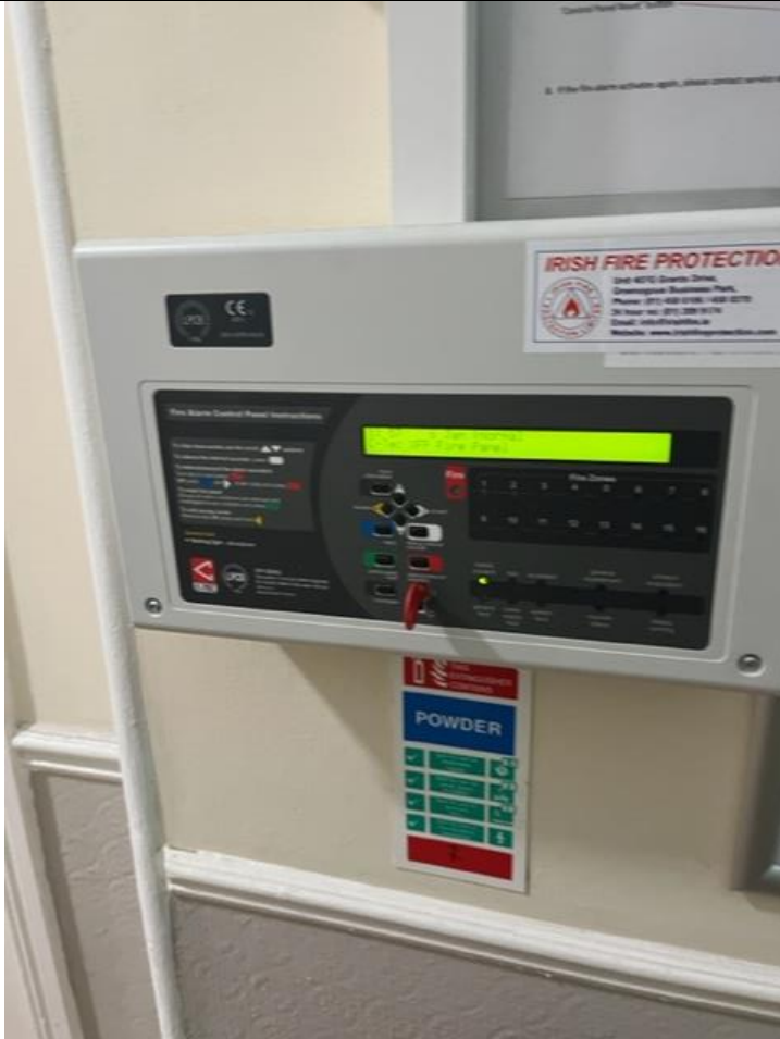
Fire Alarm Panel
