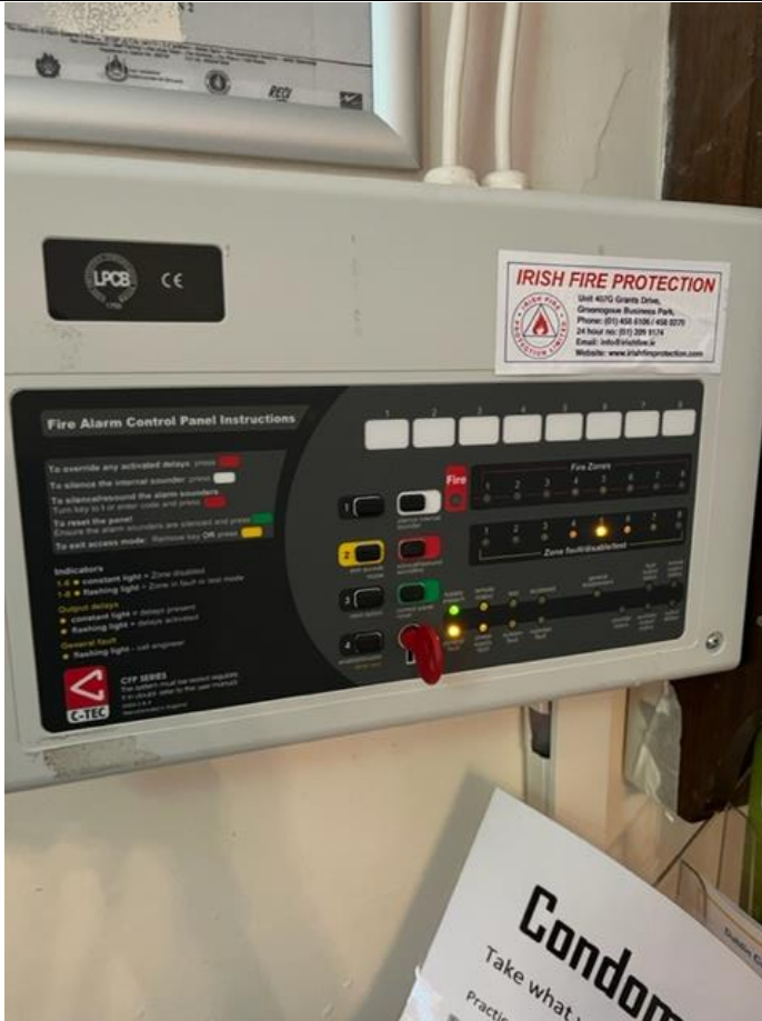
Fire Alarm Panel Showing Fault
